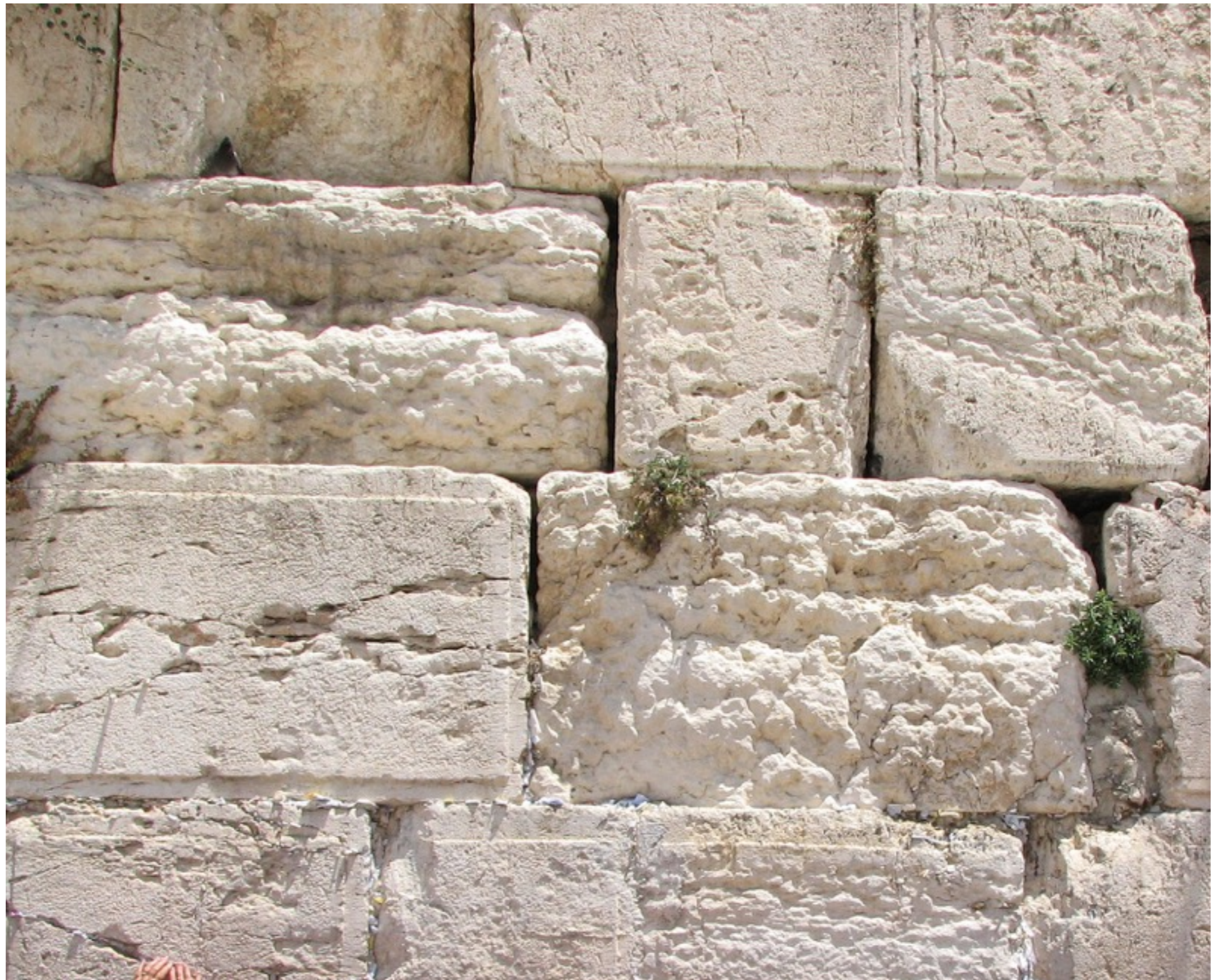
Ashlar limestone construction of the Western Wall of the Temple Mount from the Herodian period
